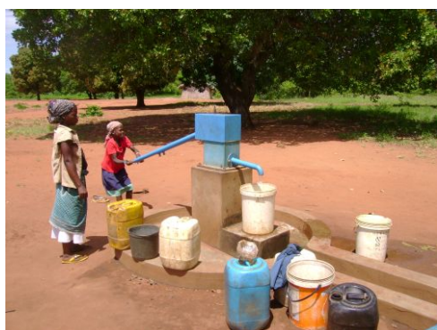
Bluepump at 65m deep on rehabilitated borehole, Unicef project Mozambique
